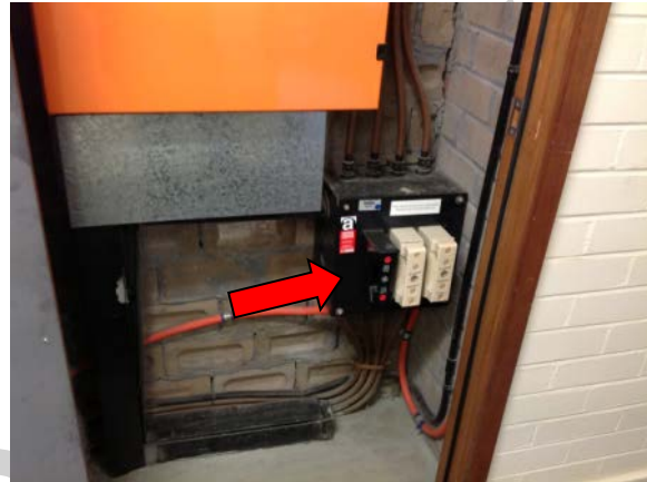
Figure 8: Kensington Campus, Morven Brown Building, Ground Level, Room GQ4, Electrical Distribution Board – Compressed bituminous electrical panel
