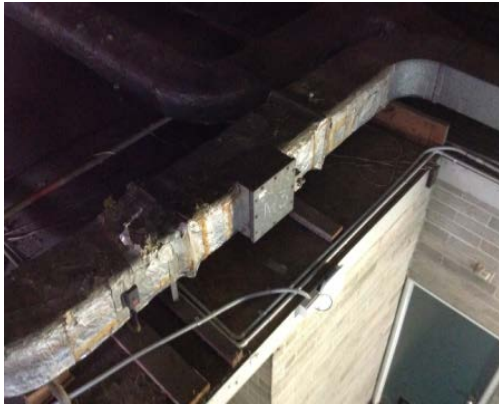
Figure 10: Randwick Campus, Building R9 (Tram Shed), Ground Level, Room G20, on top of ceiling – asbestos containing millboard insulation
