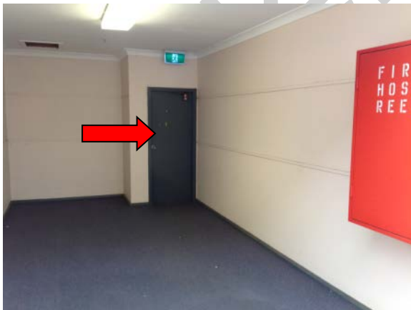
Figure 11: Randwick Campus, Building R9 Tram Shed, Mezzanine Level, Room MQ2, Stairwell – fire door core
