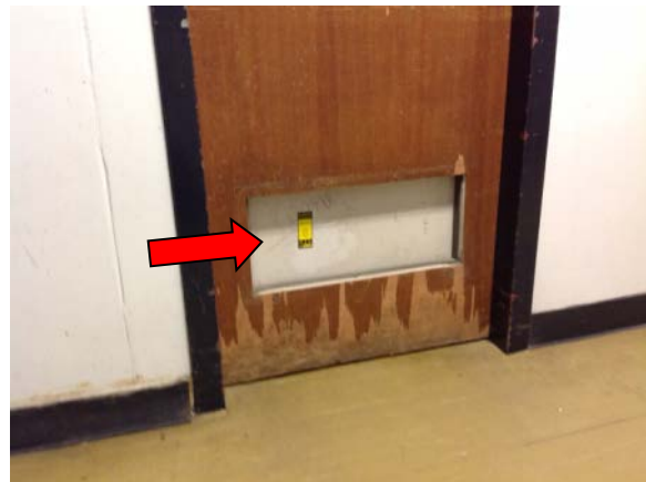
Figure 12: Kensington Campus, Building D26 Biological Sciences, Level 3, Room 340 – fire door core
