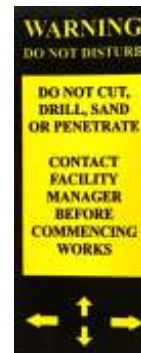
Figure 2: asbestos warning labels used at UNSW
